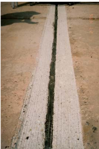
Figure 13: Expansion joint after milling, before placement of the sealant and the rubber sheet.
