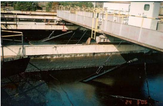
Figure 5. Oil and grease deposits on the surface of concrete tanks
