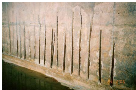
Figure 4. Delaminating concrete due to corrosion of reinforcing steel
