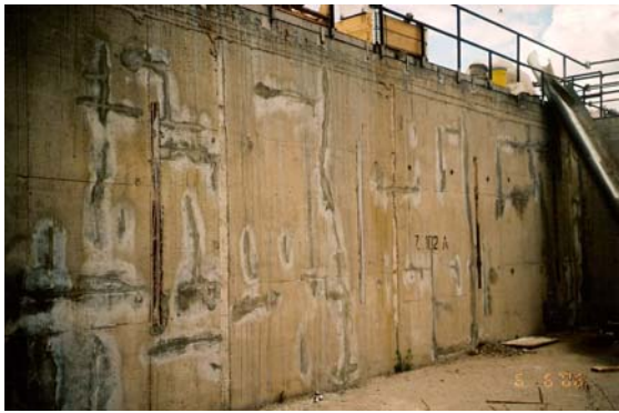
Figure 11. Cracks filled with fibre reinforced mortar bonded with polymer modified cement slurry to the polyurethane seal
