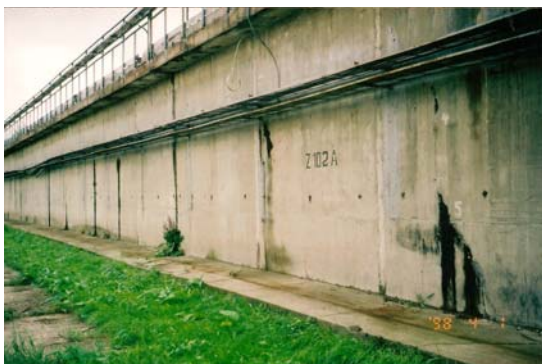
Figure 3. Leaks in concrete tanks
