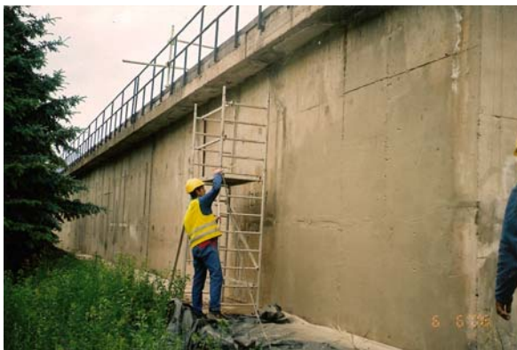
Figure 17. Application of one component polymer modified cement coating to the exterior of the tank
